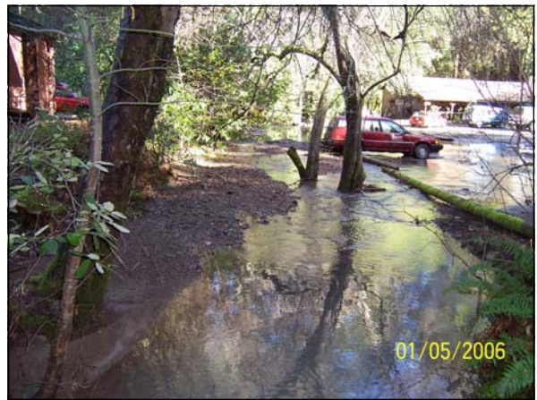
Undersized culvert has plugged and is now flooding the road and parking lot.
